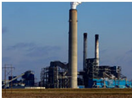
Coleman power plant Source: Big River Electric Corp.
